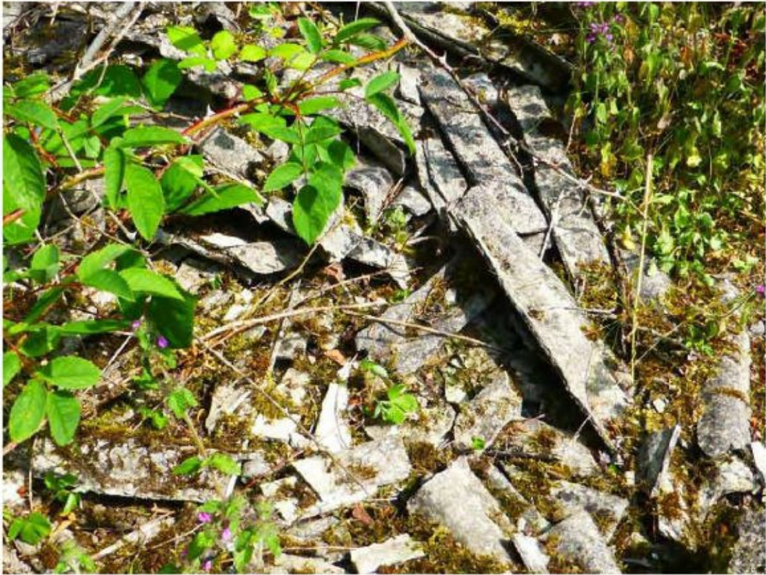
Recently fly-tipped material. Includes asbestos roof sheeting. Resulting from Estate maintenance activities?
